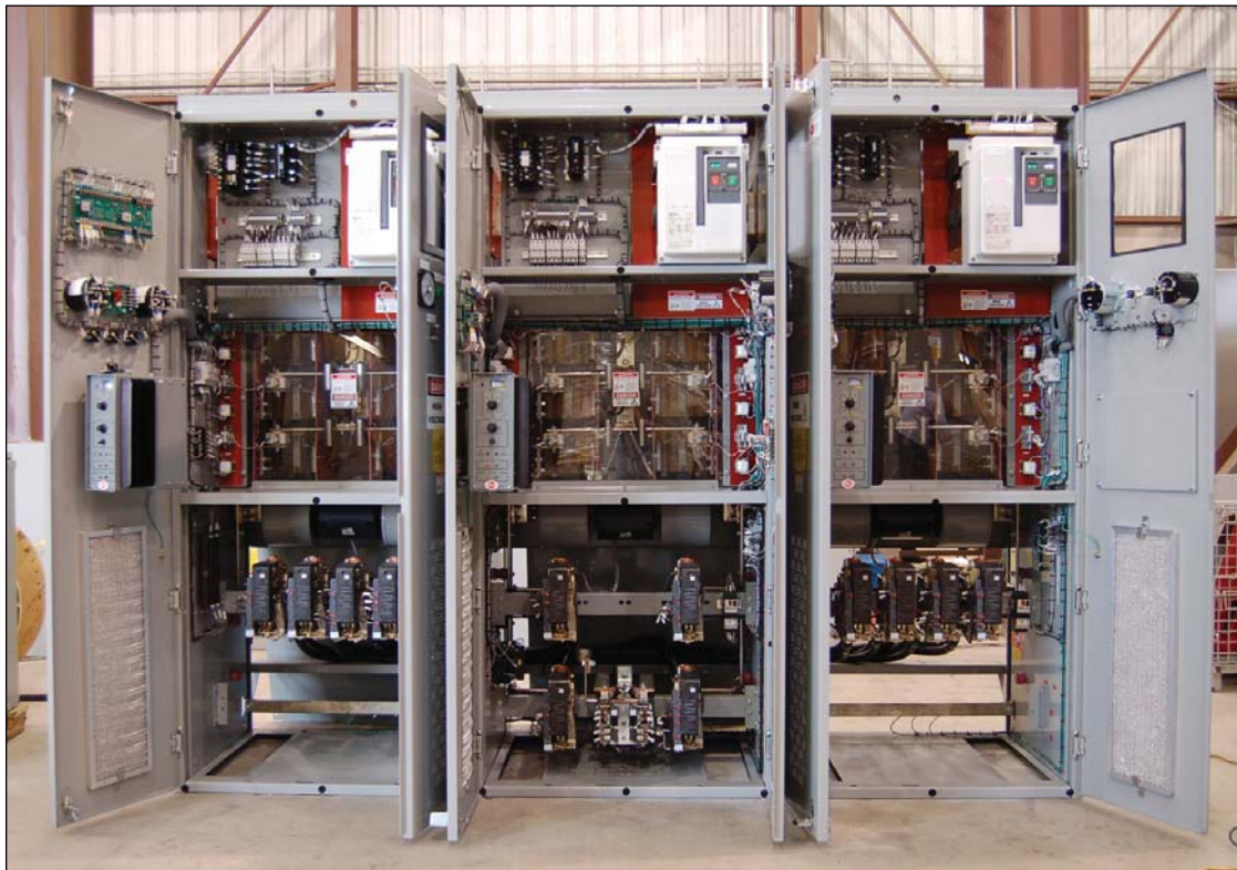
This AETI DC SCR drive system is typical of equipment used on drilling rigs to power drawworks, mud pumps, rotary, or top drives. This power gear is similar to what will be manufactured through the new AETI alliance in Brazil (Fig. 2; photo from American Electric Technologies Inc.).
